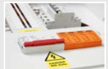
SPD mounted beside main switch
